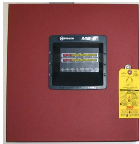
Figure 24: Fire Alarm Control Panel
