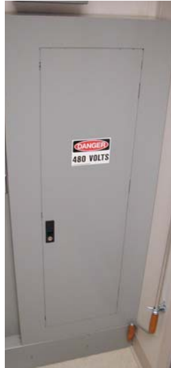
Figure 32: 480V AC Electrical Panel
