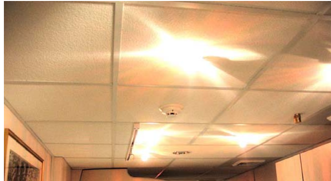
Figure 55: Scan Room Lighting
