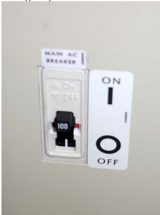
Figure 5: Cryogen Compressor Switch
