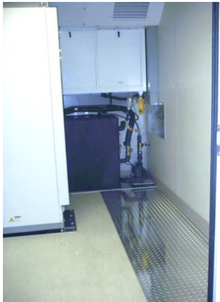
Figure 6: Equipment Room Overall
