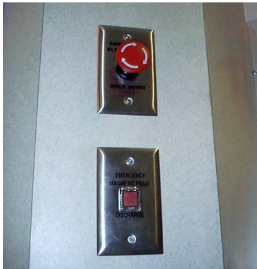
Scan Room E-Stop and Magnet Quench Controls
