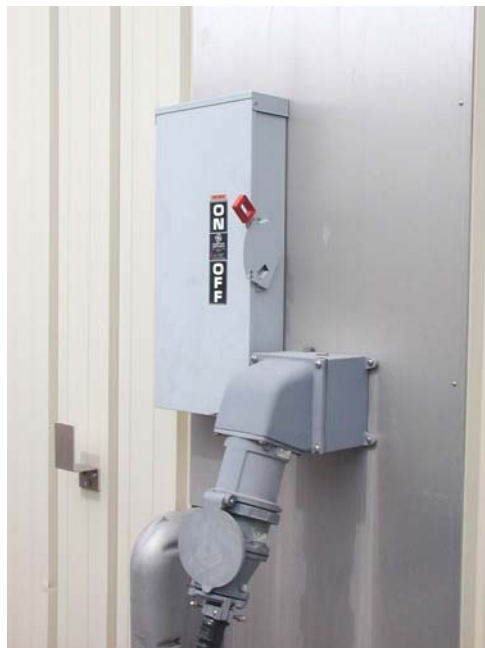
Figure 33: Shore Power Connection
