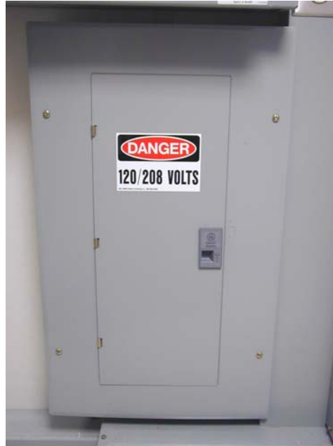
Figure 31: 120/208V AC Electrical Panel
