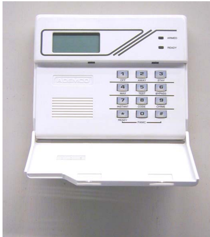
Figure 46: Intrusion Alarm Keypad
