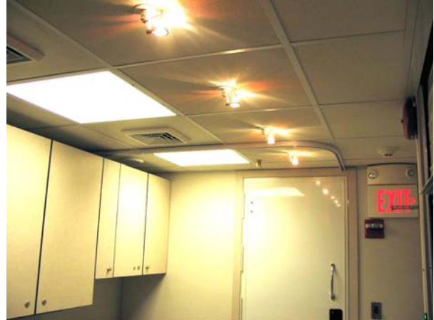
Figure 54: Control Room Lighting
