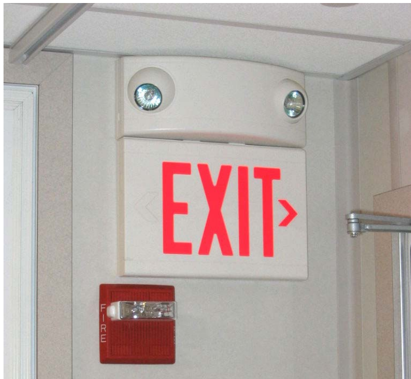
Figure 49: Emergency Dual Beam Lighting
