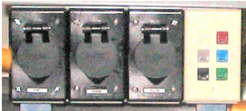
Figure 14: Phone & Data Line Connections
