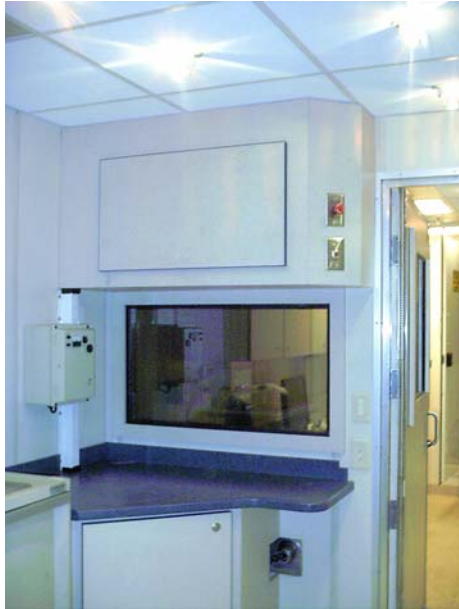
Scan Room Lighting and Magnet E-Stop & Quench Controls
