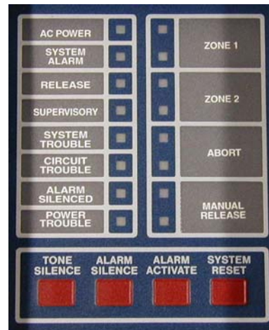
Figure 26: Fire Suppression Components
