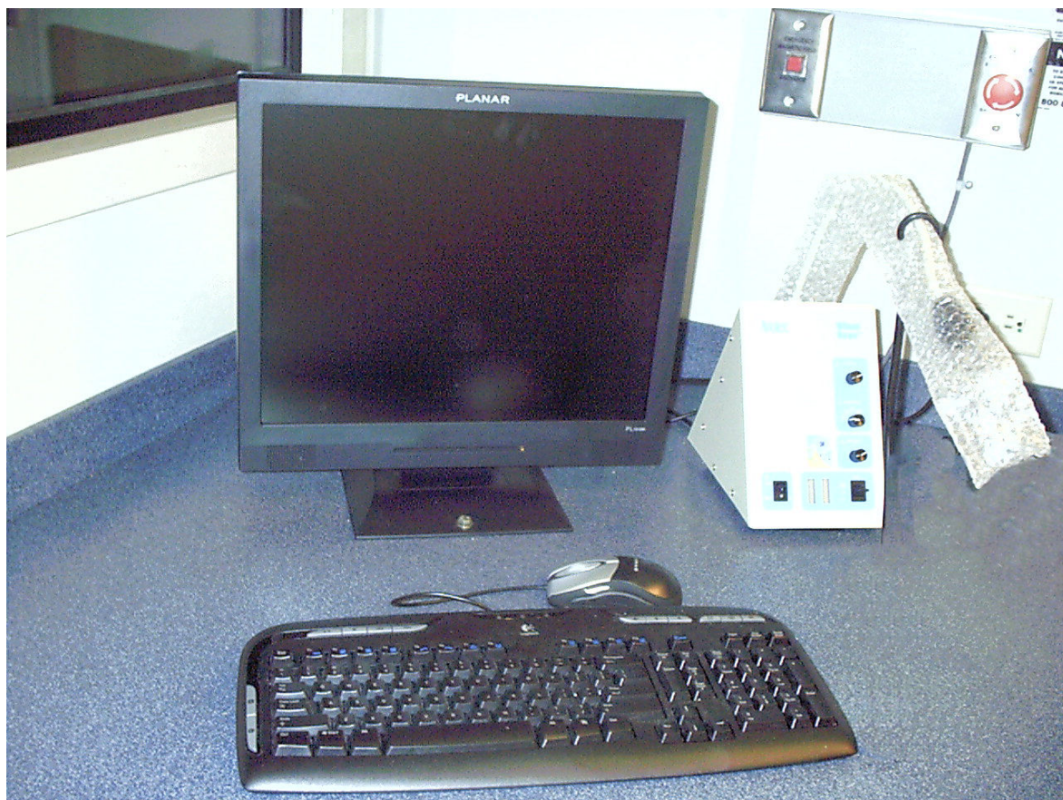
Figure 4: Control Room Overall
