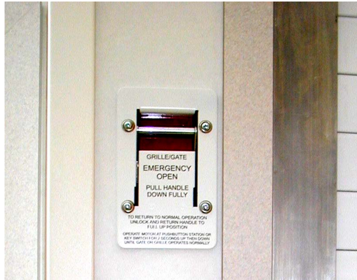
Figure 29: Roll Door Emergency Release
