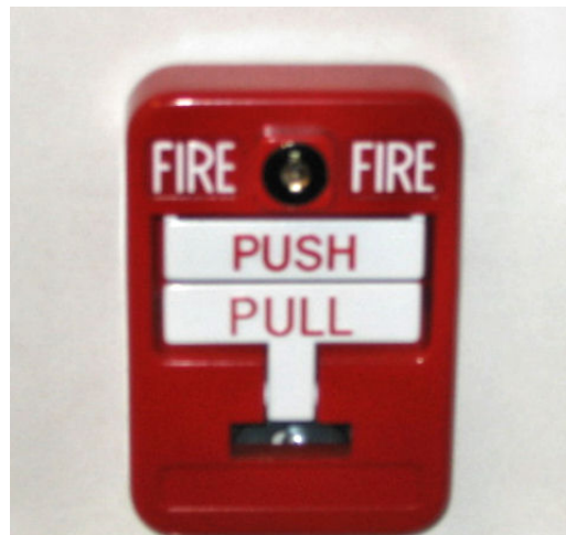
Figure 25: Fire Alarm Pull Station
