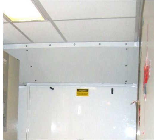
Figure 53: Equipment Room Lighting
