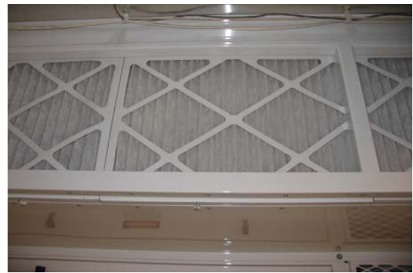
HVAC Filter Access
